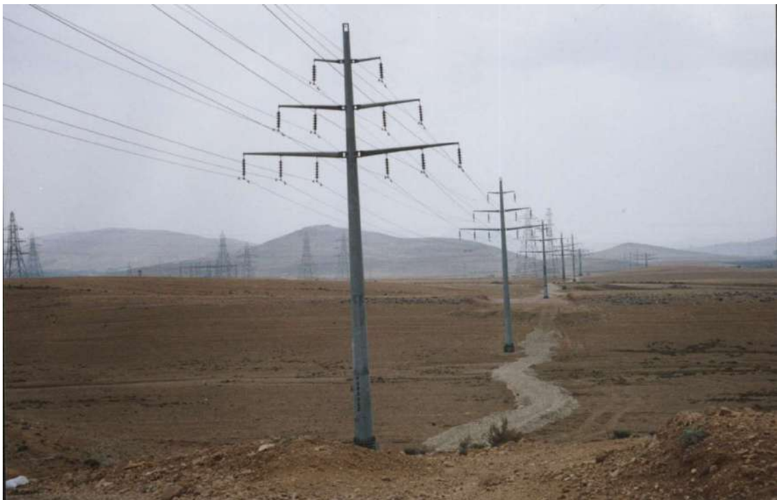
Sadra-Gholestan 66kv Four-Circuit Line in Shiraz
