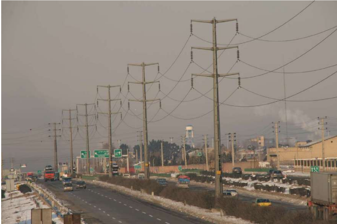
Makhsos Road 63kv D.C. Line in Tehran
