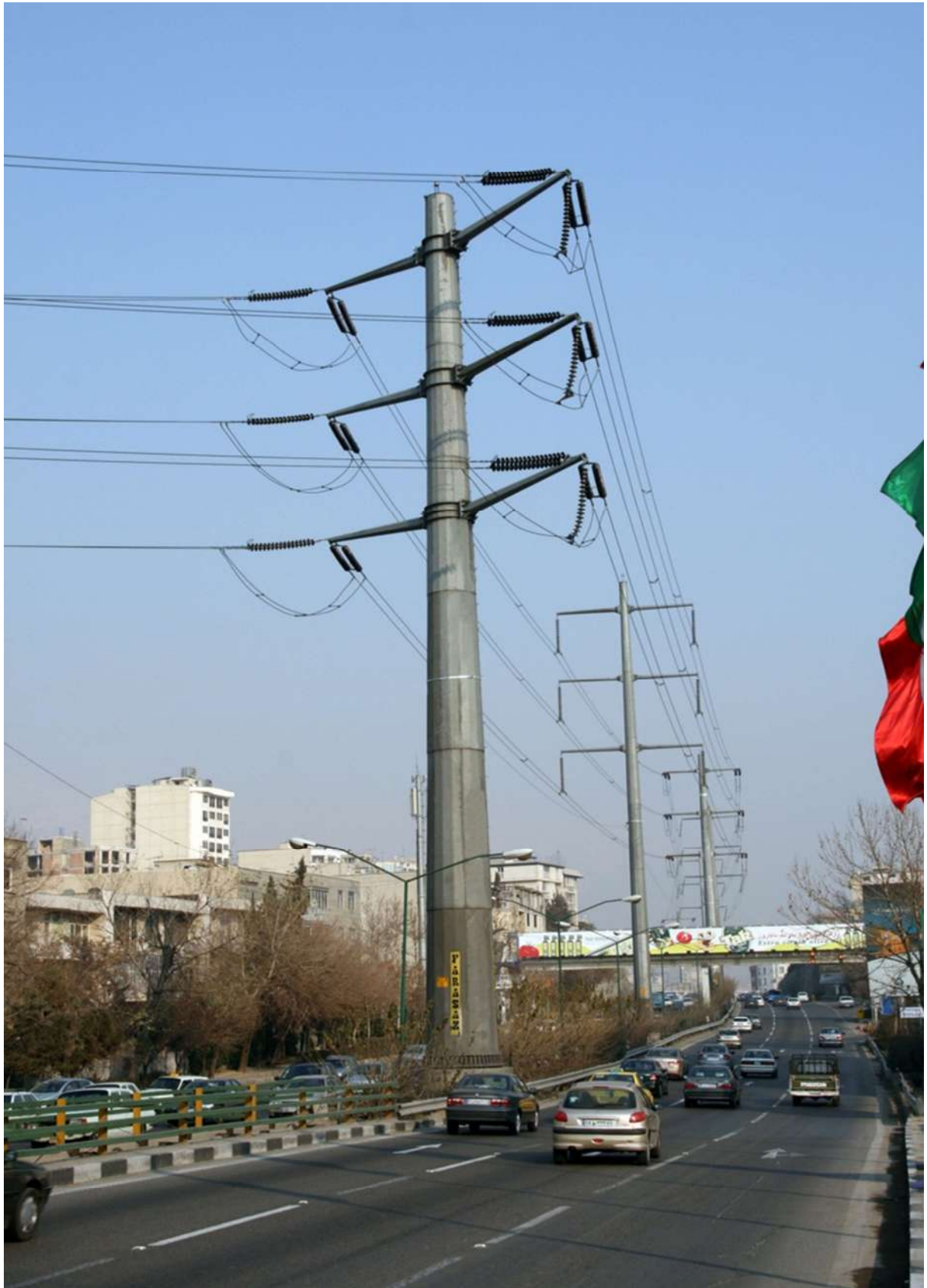
۲۳۰ kv Overhead Line in Tehran (Qeytariyeh)
